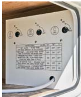
Water Command Center
